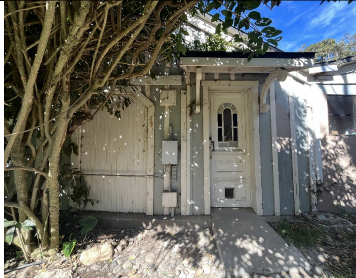
Close up of Entry on South Elevation (note turn of the century detailing)
